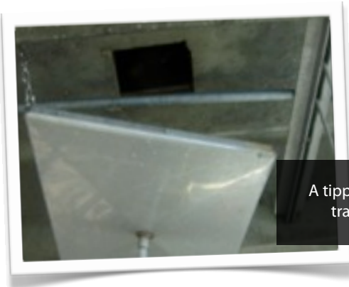
Drip pan with a plugged drain is full of water.
